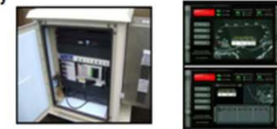
Alarm Panel & Display
